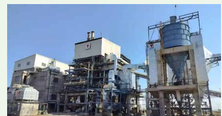
A 6.5 MW cogeneration plant for a manufacturer of ethyl alcohol, grain distillate, and DDGS in Bundi, Rajasthan
