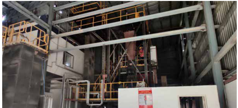
Green steam boiler plant under the build-own-operate model
