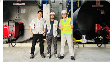
Thermax installs Shellmax Global 4 TPH boiler for a textile greenfield project in Ninh Thuan, Vietnam
