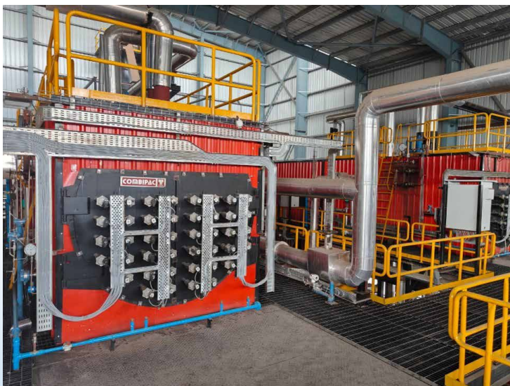
Green steam boiler plant near Mysore, Karnataka
