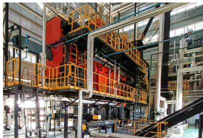
The 6 TPH UltraPac boiler at a chemical manufacturing facility at Kurkumbh, Maharashtra
