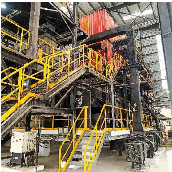
A 16 TPH green steam boiler plant at Mandideep, Madhya Pradesh
