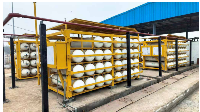
The first batch of bio-CNG cascades being dispatched
