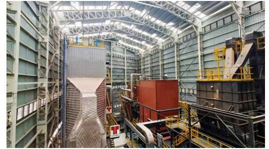
The 30 TPH biomass-based green steam boiler plant commissioned with G+1 configuration
