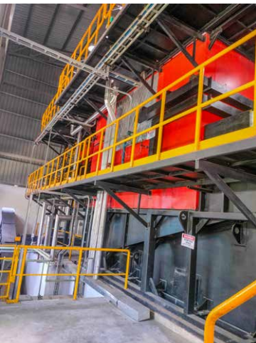
A 10 TPH biomass boiler installed at Chennai
