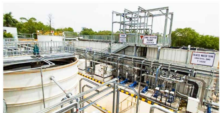
Site image of the sewage treatment plant installed at Gurugram, Haryana
