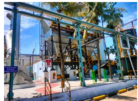
The green steam boiler plant supplied under the build-own-operate model
