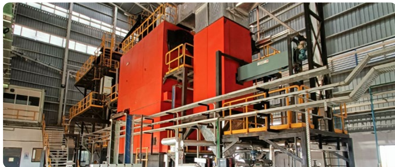
TOESL partnered with a leading specialty chemicals company, marking their third collaboration for green steam supply under the build-one-operate (BOO) model
