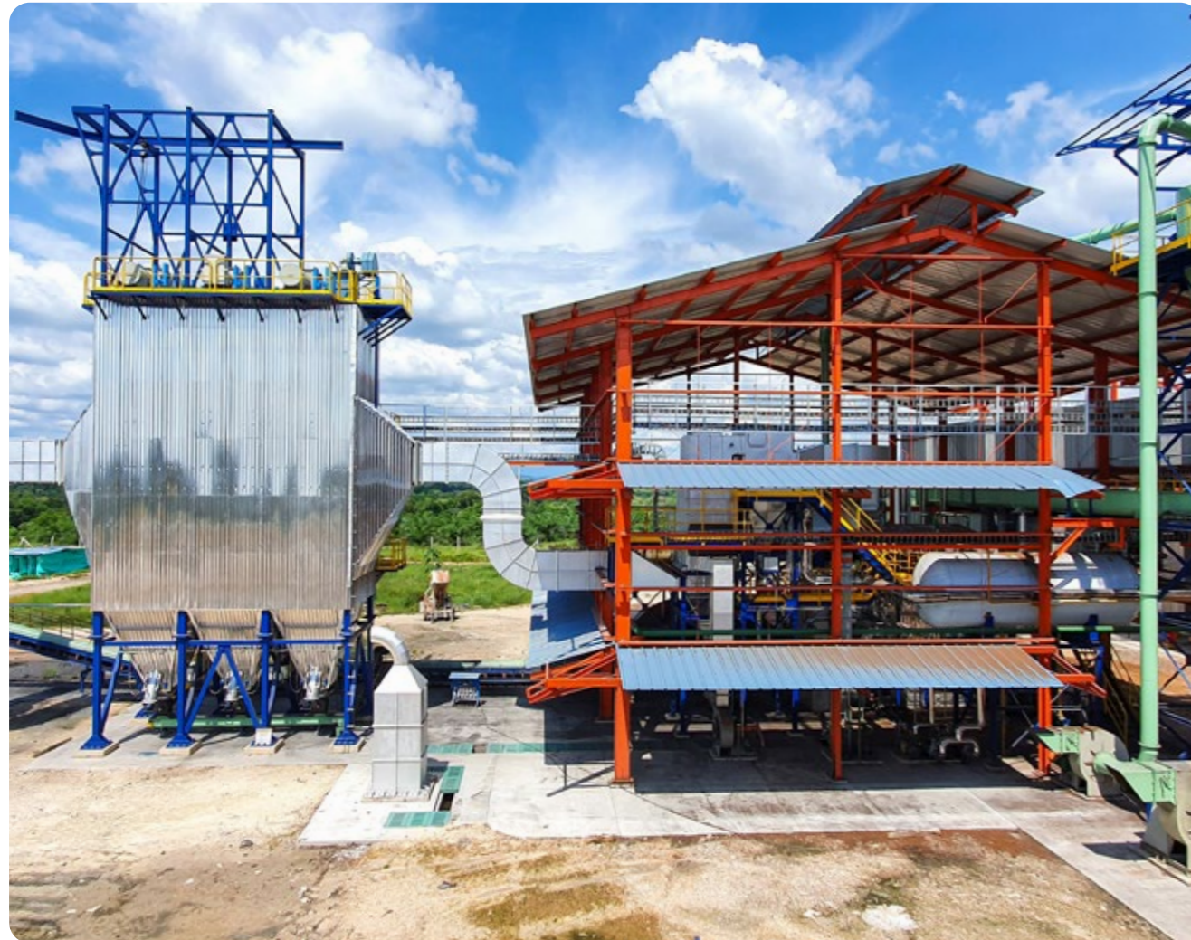
An electrostatic precipitator (ESP) commissioned for a leading palm oil producer in Columbia. The ESP is for a biomass-fired boiler that uses palm shell and fibre as its primary fuel.
