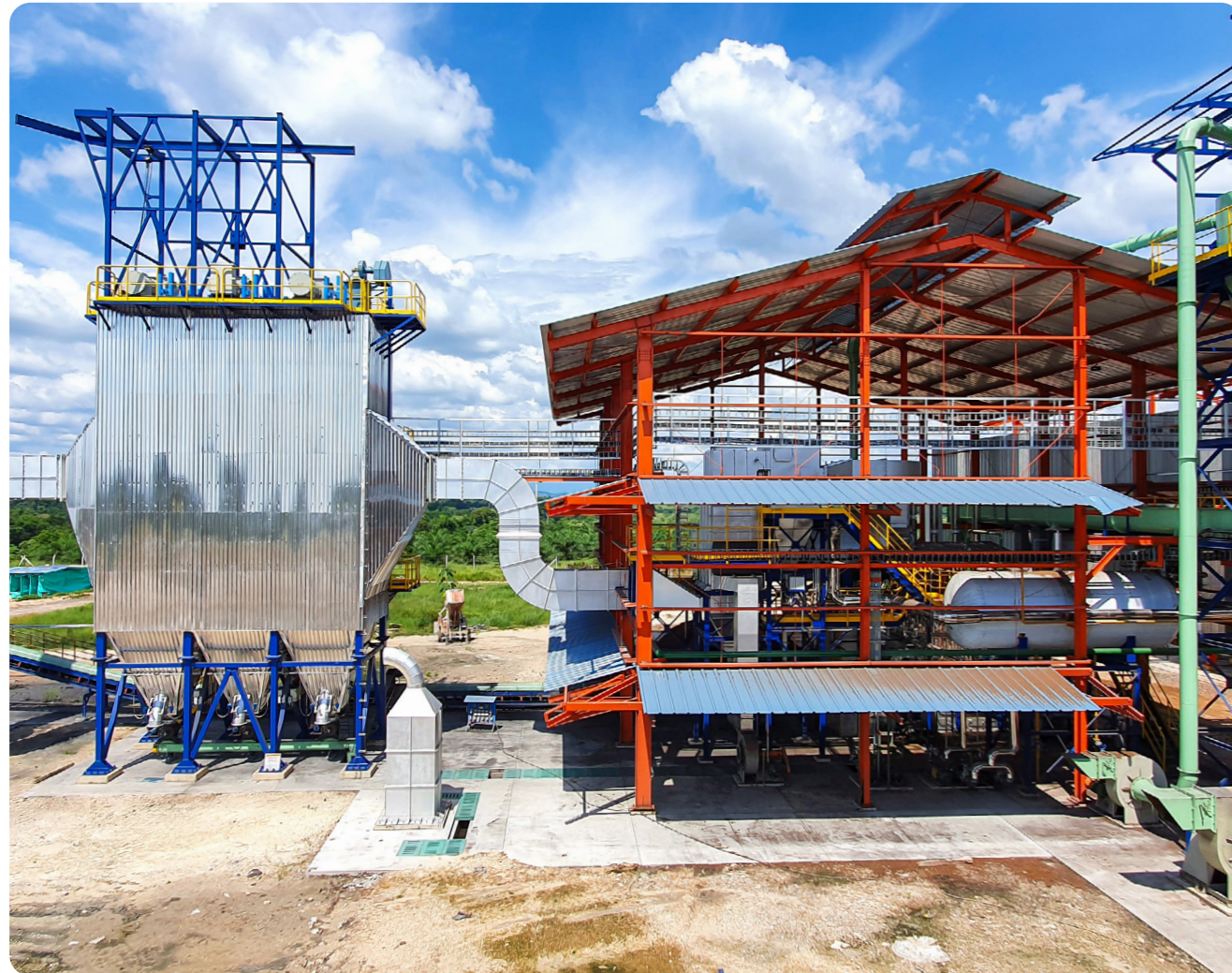
An electrostatic precipitator (ESP) commissioned for a leading palm oil producer in Columbia. The ESP is for a biomass-fired boiler that uses palm shell and fibre as its primary fuel.
