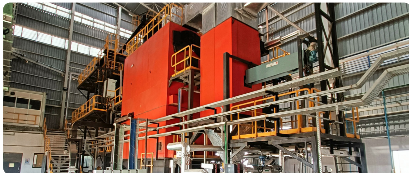
TOESL partnered with a leading specialty chemicals company, marking their third collaboration for green steam supply under the build-one-operate (BOO) model
