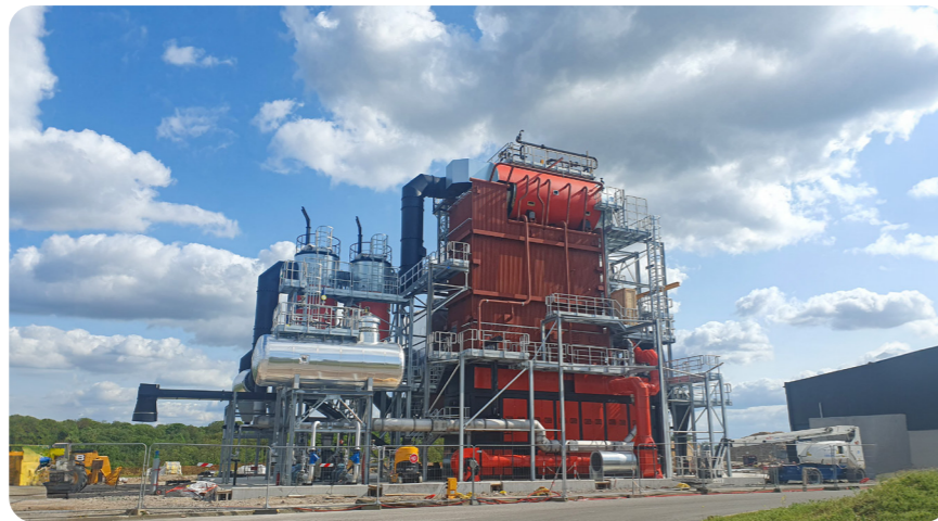
The 26 TPH boiler supplied and installed by Danstoker for a dairy company in France
