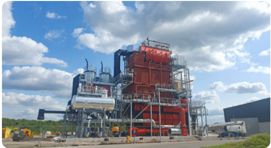
The 26 TPH boiler supplied and installed by Danstoker for a dairy company in France
