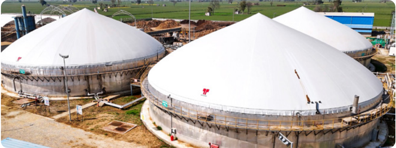
A site image of our bio-CNG plant in Dhuri, Punjab
