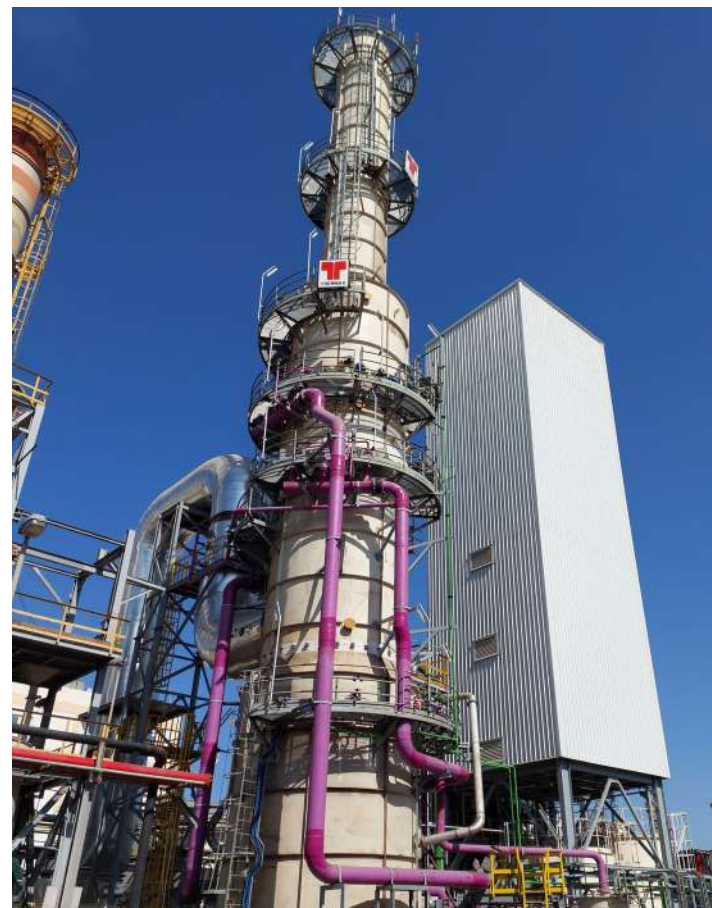
A state-of-the-art flue gas desulphurisation (FGD) system delivered to a prominent sugar refinery in Saudi Arabia
