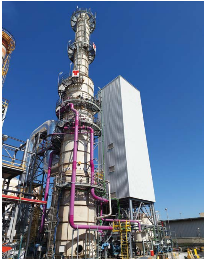
A state-of-the-art flue gas desulphurisation (FGD) system delivered to a prominent sugar refinery in Saudi Arabia
